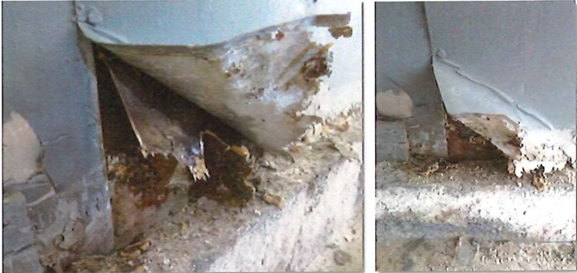
When the metal wall finish is peeled away, evidence of rotting sill plates can be seen.
