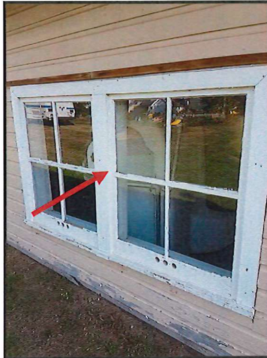
FIGURE 7: WHITE LEAD-BASED PAINT ON WOOD WINDOW FRAME, NW CORNER OF BUILDING EXTERIOR
