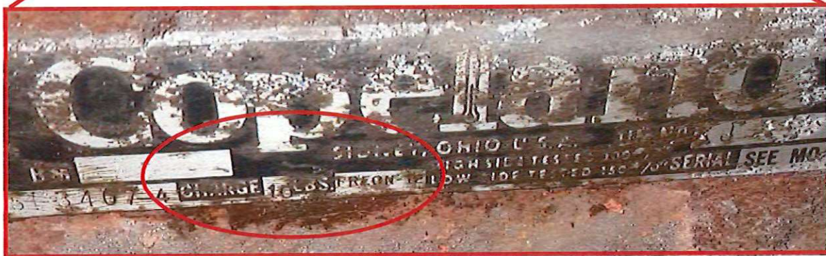
FIGURE 14: AIR CONDITIONING COMPRESSOR WITH CFC-CONTAINING REFRIGERANT (10 LBS OF FREON-12) IN MACHINE/ELECTRICAL ROOM
