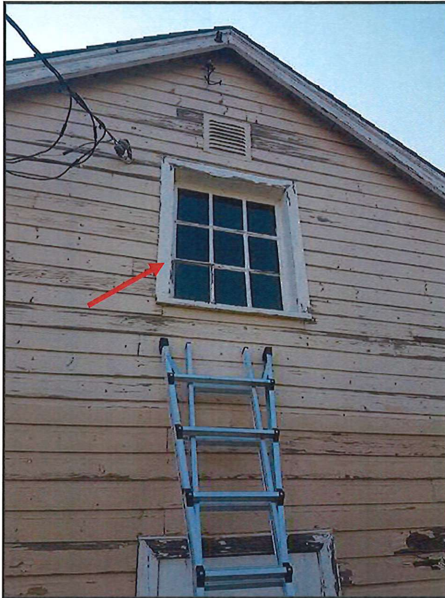
FIGURE 10: WHITE LEAD-BASED PAINT ON WOOD WINDOW FRAME, NORTH SIDE OF BUILDING EXTERIOR
