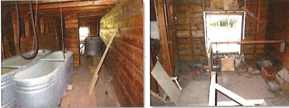
The attic flooring at the rear of the building is made of wood planks.
