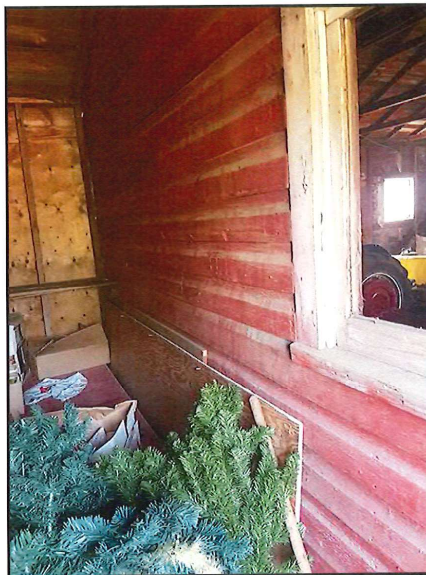
FIGURE 13: RED LEAD-BASED PAINT ON WOOD WALL BOARDS, NORTH SIDE OF GARAGE INTERIOR, DIVIDING WALL
