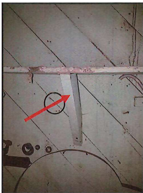
FIGURE 5: WHITE LEAD-BASED PAINT (BENEATH GREEN PAINT) ON WOOD SHELF SUPPORT, HALLWAY ADJACENT TO TANK ROOM
