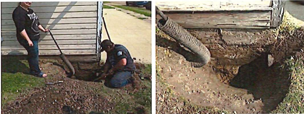
Digging in the SW corner revealed what appears to be a 24" deep grade beam on piles
