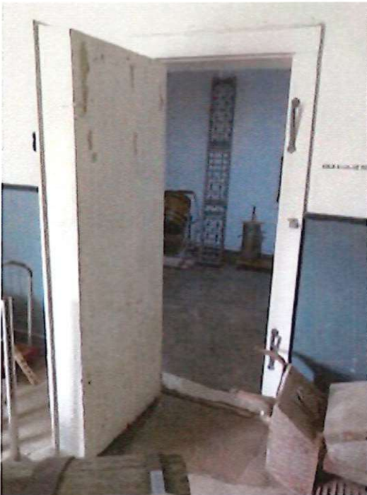
The insulated cooler room door – good condition
