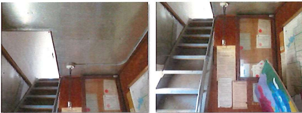
The ceiling of the attic access office is unpainted metal. The walls are varnished plywood.
