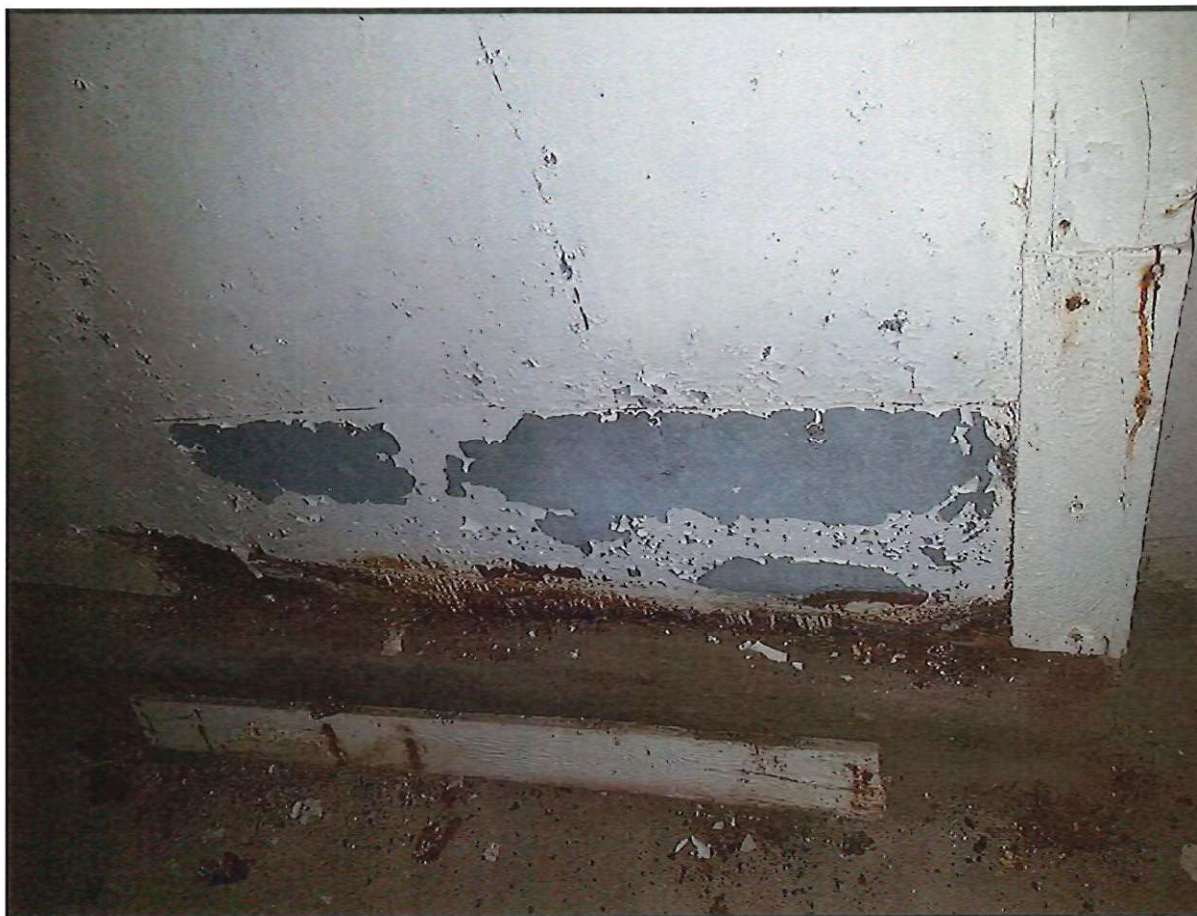
FIGURE 15: WATER DAMAGED METAL WALL SHEETING AND SUSPECTED MICROBIAL GROWTH ON WOOD BASEBOARD AND BEHIND METAL SHEETING ON EAST WALL OF ICE MAKER ROOM
