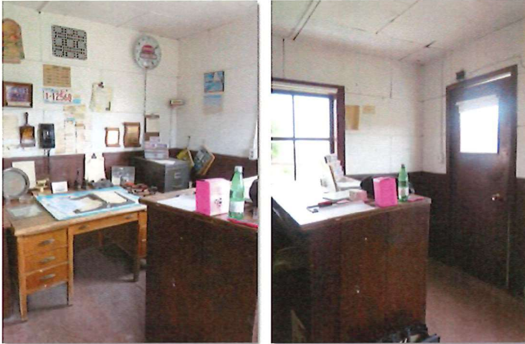
The office walls and ceiling are clad in painted Tentest fibreboard, commonly used in the 1950s as a wall finishing material, are in good condition.
